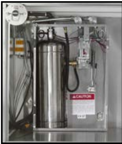
ANSUL canister inside base cabinet
